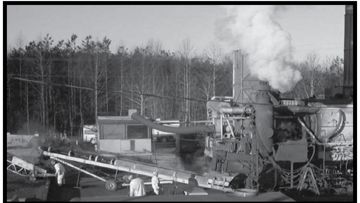
PCB and dioxin contaminated soils were treated with a high capacity indirect thermal desorption unit for the Warren County Landfill cleanup.
